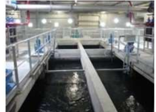
Granulated Activated Carbon filters
